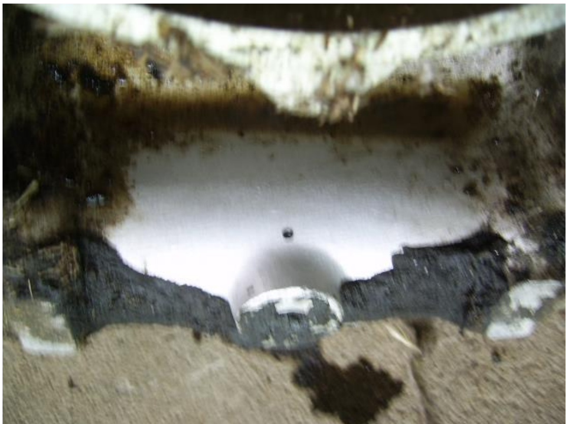
Figure 2 Close up of said hole
