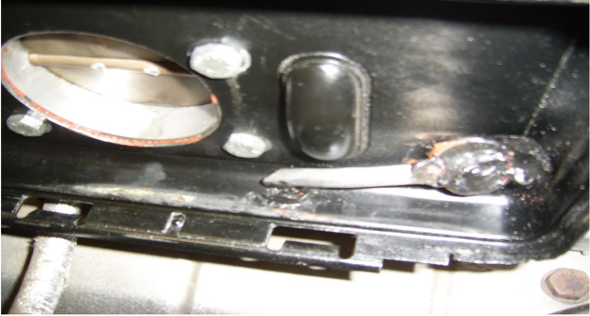
Inside the LH air filter showing the dist cap vent pipe
